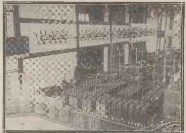
A view of part of the transmitting hall at the Nauen station. Note the large banks of condensers in the foreground.
