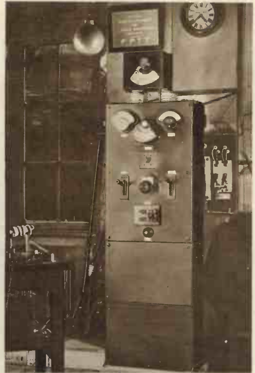
Fig. 1.—The control switchboard for the generator system.
