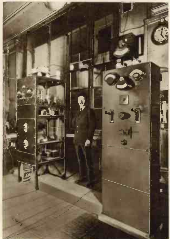
Fig. 8.—The control switchboard for the transmitter is seen on the left of this photograph.
