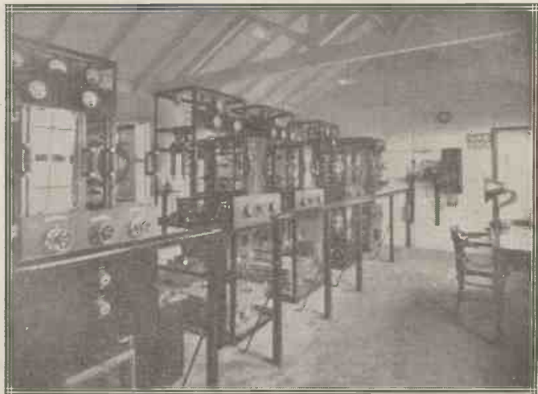
This photograph shows the Marconi Transmitter at the Belfast Station, which was opened recently.
