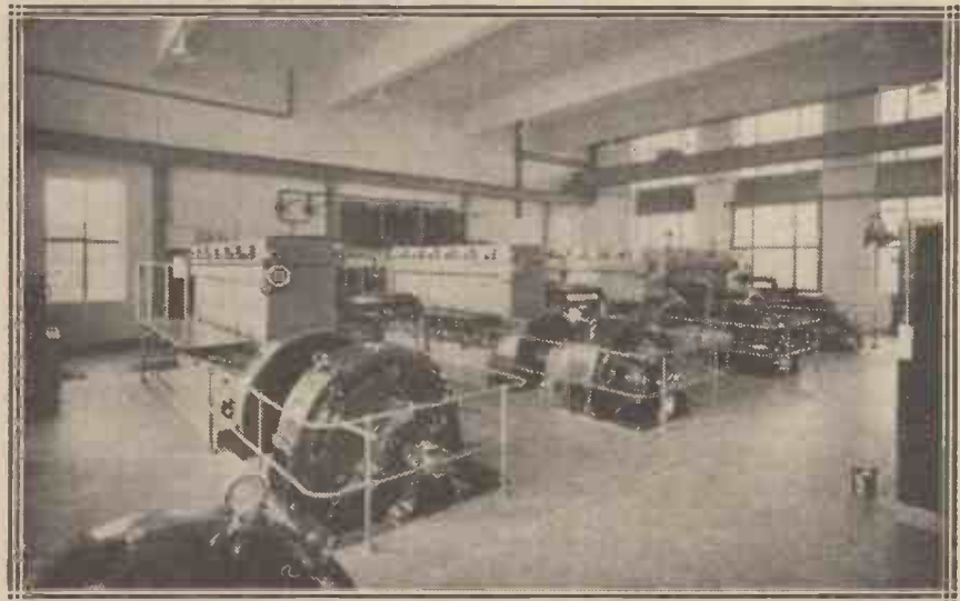
ONE OF THE LATEST WORLD VOICES, the West Regional transmitter at Washford Cross in Somerset. This is the power house, with its four Diesel engines and generators.
