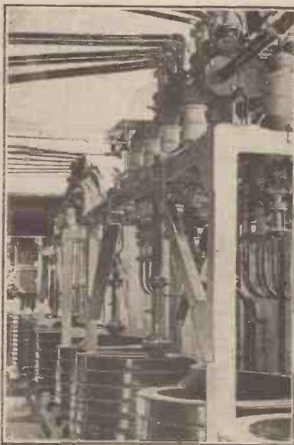
“Even now, with the high-power stations pumping out 100 kilowatts or more, the selection of daylight-range foreigners is very limited,” writes the author of this article. Here is the massive control gear for the valve-cooling plant at one of the powerful German stations.
