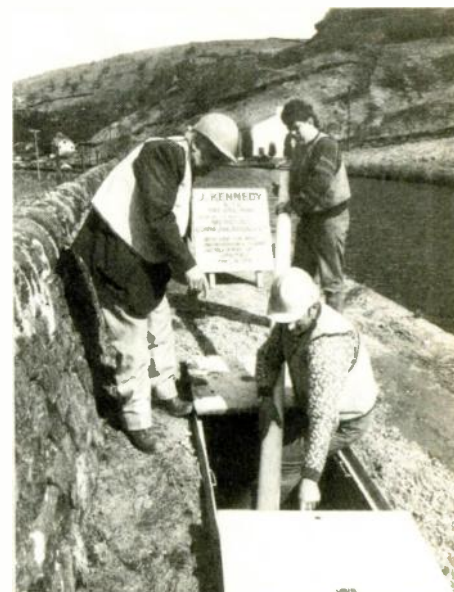
190-year-old Rochdale canal is once again to become part of a national communication network. But this time telephone traffic rather than cargo barges will be carried. It was actually the ease of laying the cable under the towpath that attracted Mercury Communications to link Leeds and Manchester in this way. The only hazard was discarded trolleys.
