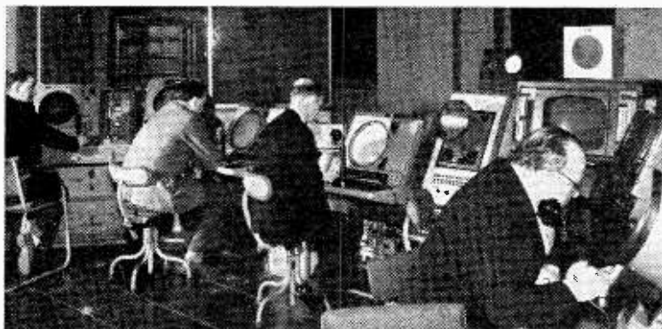
Radar Control Room. —Marconi's have supplied three complete radar installations for the new Royal Aircraft Establishment at Bedford. In this view of the control room the two operators in the centre are at the control positions of the two 10-cm sets providing high and low long-range coverage and the operator on the right is controlling the 50-cm general surveillance radar.
