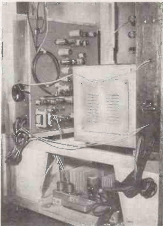
In this interior view of the receiver the delay-line cable in Fig. 2 (next page) can be seen arranged in a coil.
