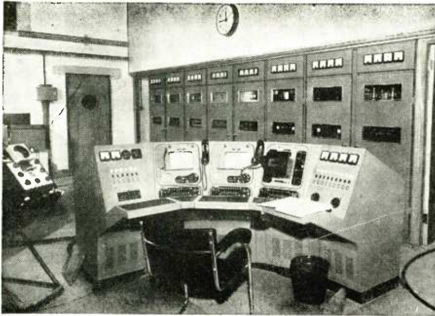
View of the vision and sound transmitters at Rowbridge with the control desk in the foreground.
