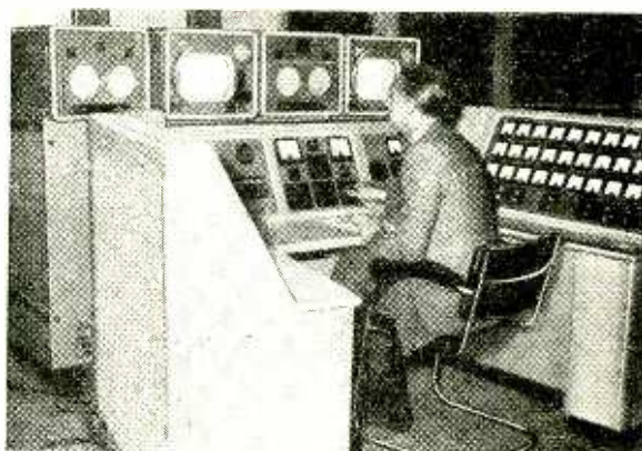
Control desk for the low-level modulation transmitter at Kirk O'Shotts.
