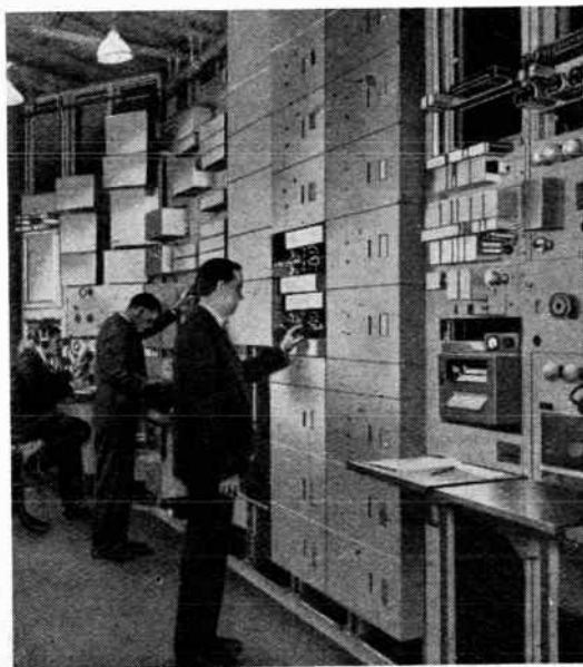
Fig. 4. New York terminus of carrier telephone system.
