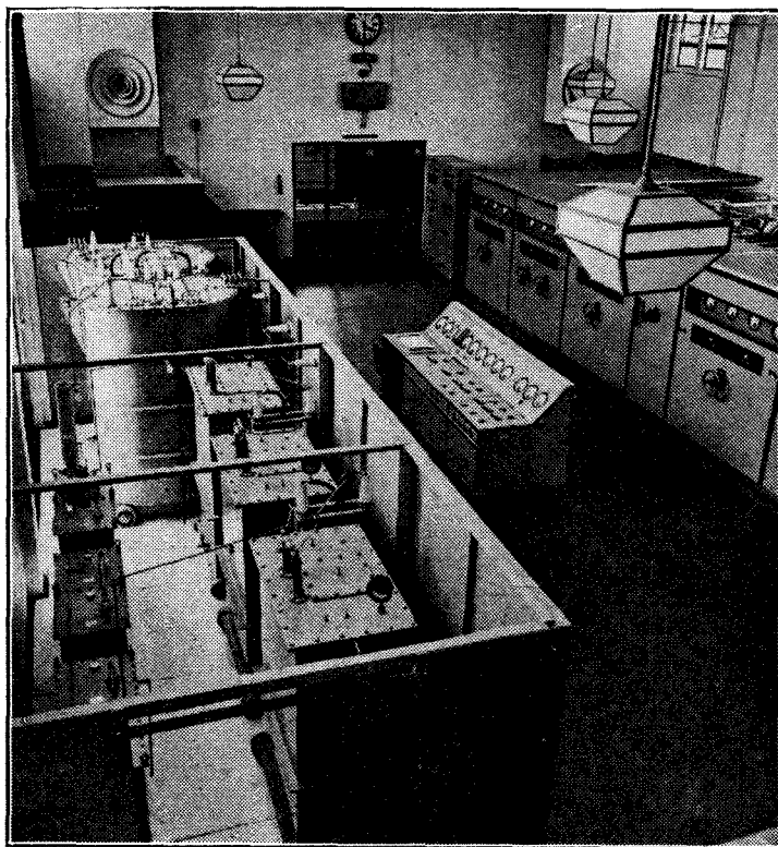
Transmitter Hall as seen from the gallery. The transmitter is on the right and the modulation transformer and plate feed reactors are in the cubicles at the left of the picture.
