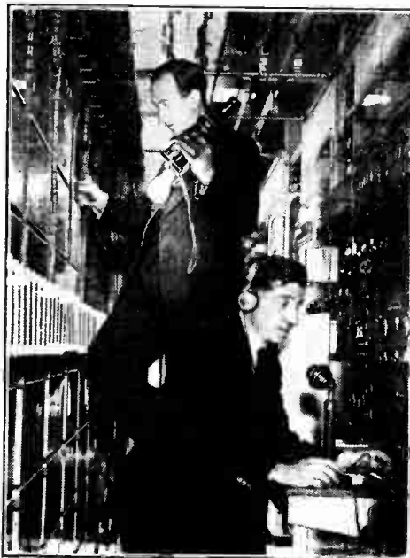
BEHIND THE SCENES. B.B.C. engineers checking amplifier performance behind one of the panels in the Control Room at Broadcasting House
