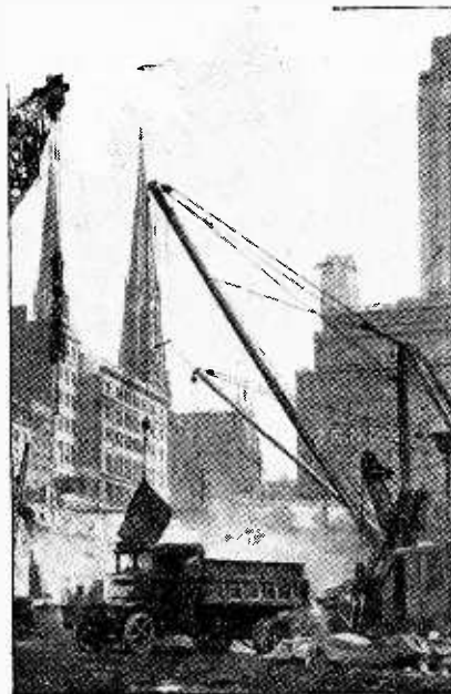
A RADIO CITY. Excavations have now begun in earnest on the site of New York's "Radio City" between Fifth and Sixth Avenues. The plans include a roof terrace and a sunk garden.
