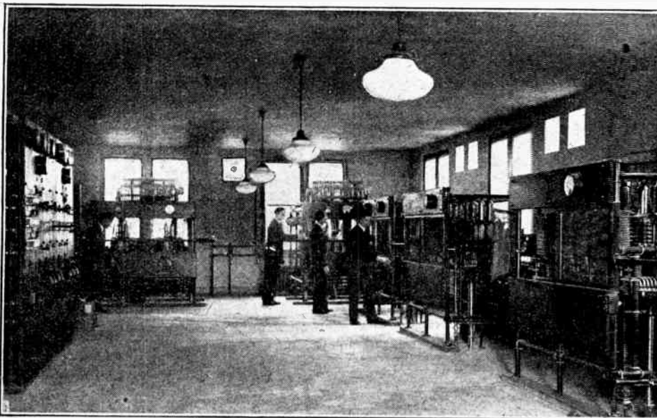
AN AMERICAN HIGH-POWER STATION. America's ambitions in broadcasting are indicated by the construction of WJZ, Bound Brook, N.J., operating with a power of 50 kW. The above photograph was taken in the transmitting room, which actually contains three 50 kW. instruments, including an emergency transmitter and a short-wave set.
