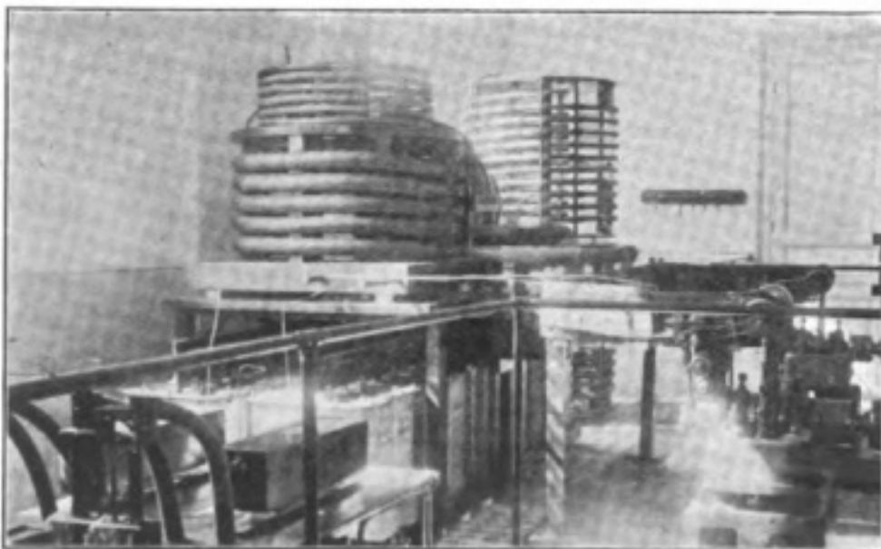
A view of the Transmitting Room showing the high-tension gear.
