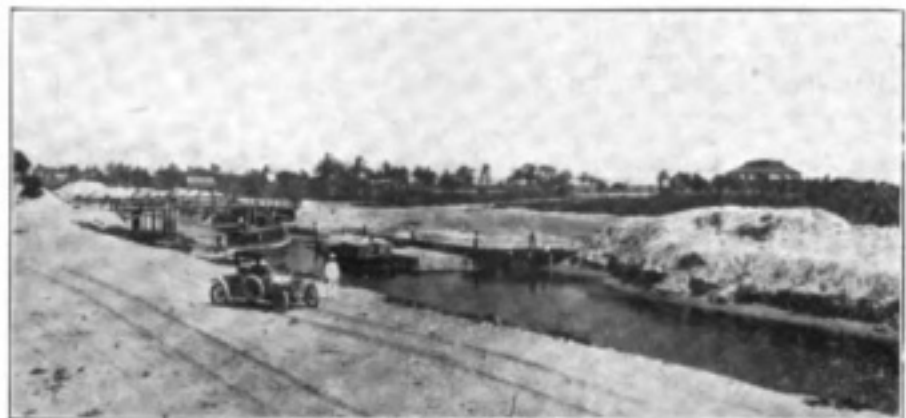
General view of the Miami Site, the towers to be built near the bridge.
