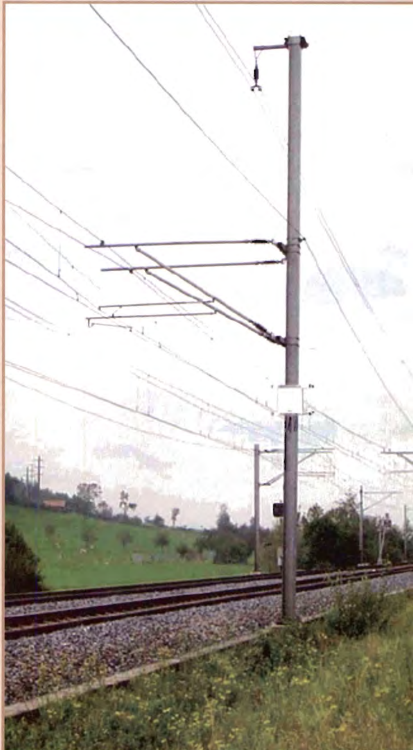
Figure 6: WLAN trackside antenna
