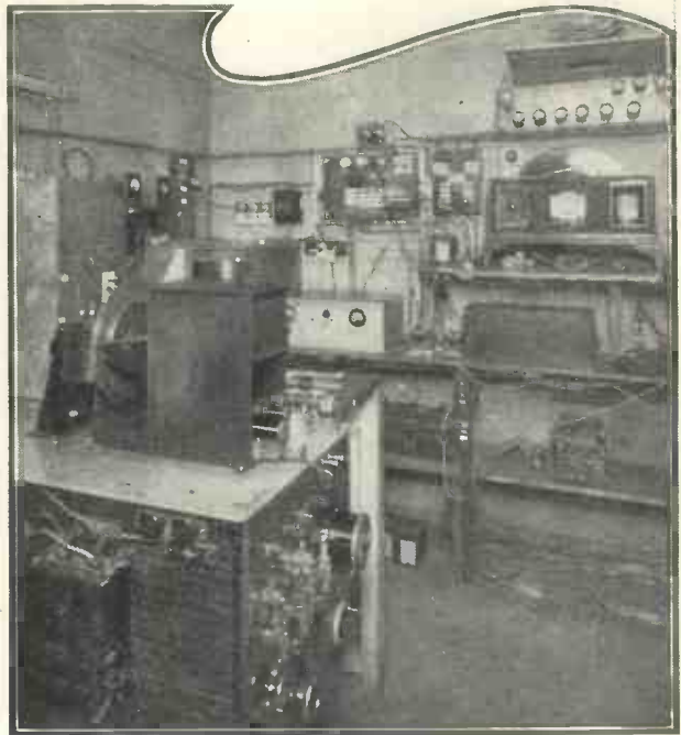
BAIRD'S OLD CONTROL ROOM
