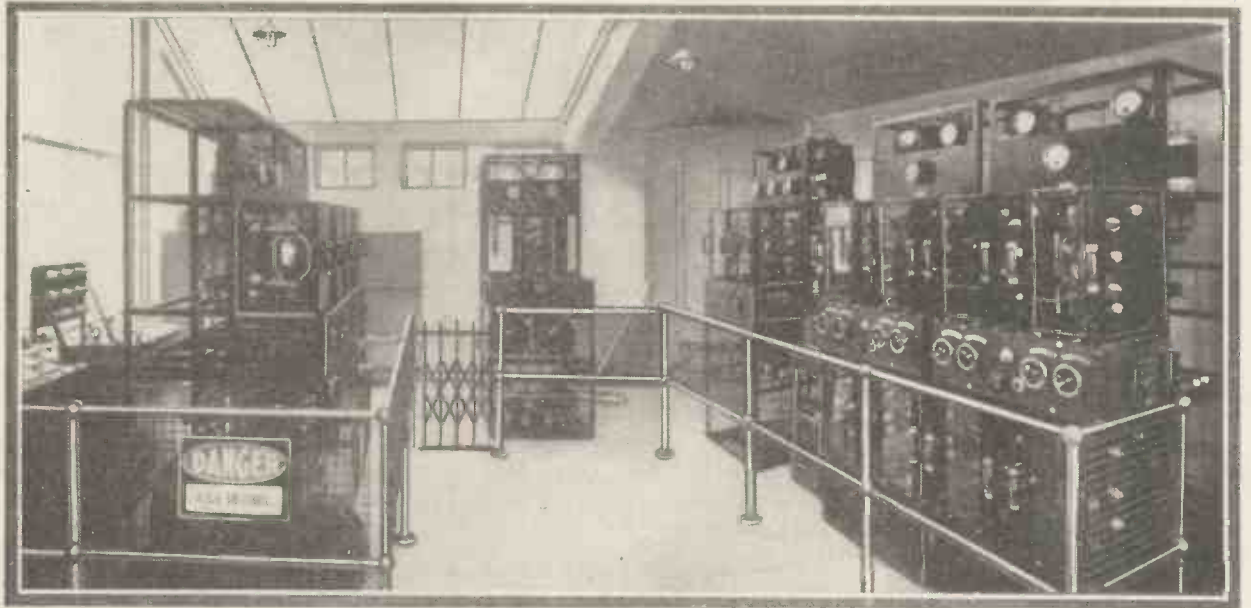
London's transmitting gear, situated on the roof of a large Oxford Street store.
