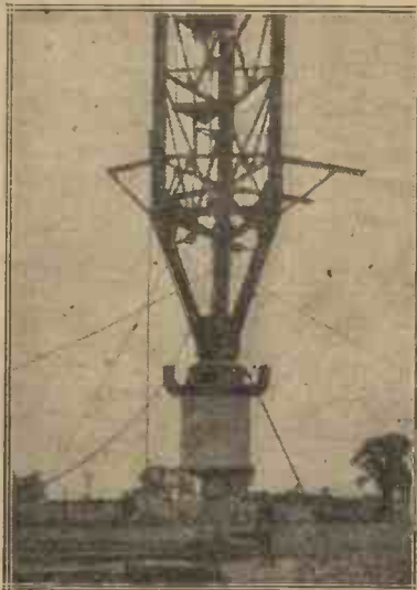
The bases of huge aerial masts are pivoted to allow the masts to sway in the wind.
