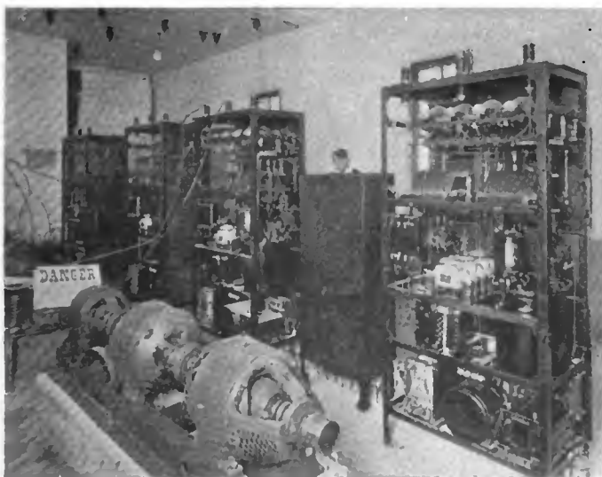
Soon to be heard on the air—the two transmitters in the little radio house on the roof of Aeolian Hall, New York City, with part of the motor-generator plant that provides power. The danger sign means what it says: current was turned on while non-electrical workmen were still on the job, and they had to be warned
