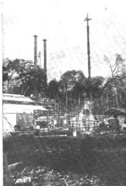
This photograph taken during the erection of the station at Porto Velho gives some idea of the type of high power equipment used in Brazil.
