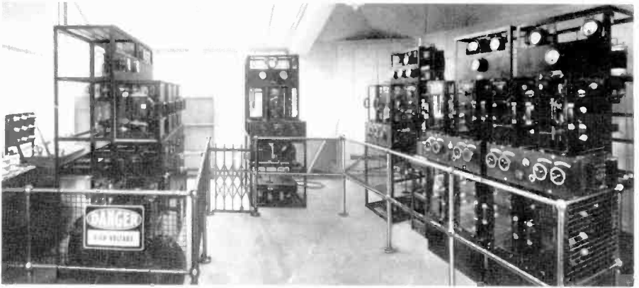
52. The refurbished 21.0 transmitter installed at Selfridges, London, March 1925. In 1929 the BBC made this transmitter available to John Logie Baird after normal broadcasting hours. These vision-only experiments with Baird's television system used just 30 lines at 12.5 frames per second.
