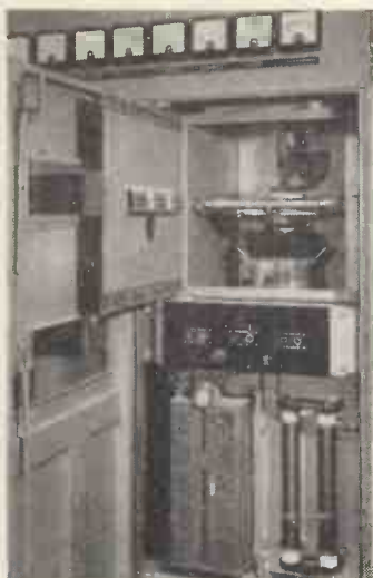
One half of the f.m. transmitter output stage, which consists of two BR128 valves in parallel in an earthed grid circuit.
