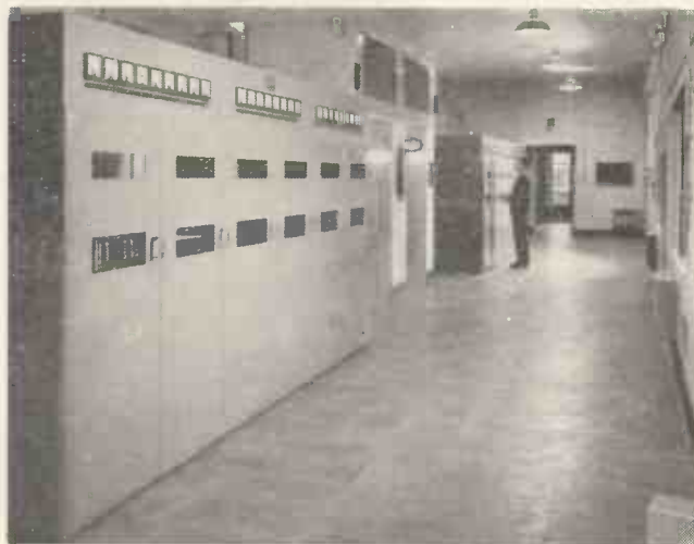
Fig. 3. Transmitter hall at Wrotham
