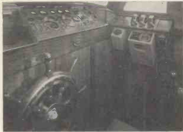
The controller and variation setter installed in the wheelhouse. The chain drive from the motor unit goes to the sprocket on the back of the wheel.
