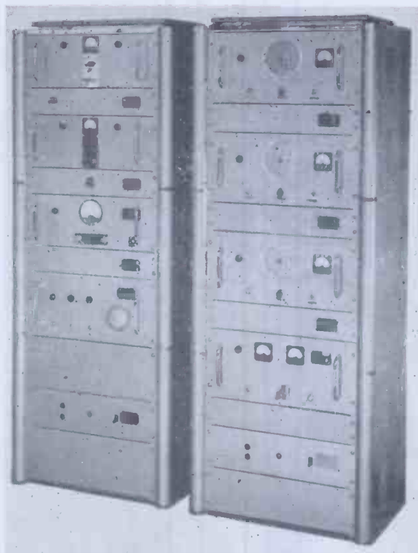
The Control Station Equipment at the Motherwell Station of the Lanarkshire Fire Authority, showing Link Transmitters and Receivers
