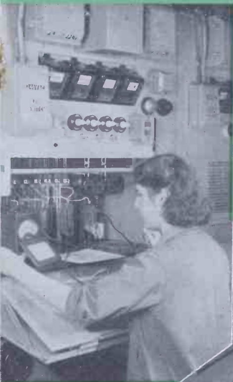
protected rack for life testing larger having inputs up to 3KV. R.M.S.
