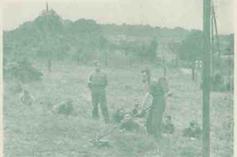
Repairing damaged wires under service conditions. The repair party are testing for mines as they go forward from pole to pole.
