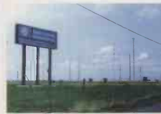
Part of the 'antenna farm' at Radio Canada's transmitter site in Sackville, NB.
