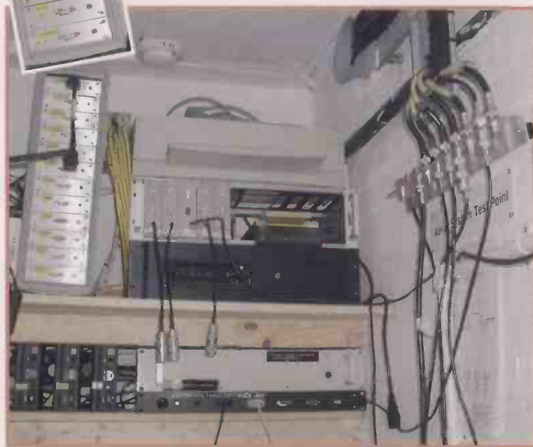
Bottom left you can see three Pye MX293s used for airband reception. Bottom right there's a GPS timing reference unit used to synchronise time on the three recording PCs. Above this is a receive distribution amplifier for airband. The centre black box is a car radio used to record on site RSL broadcast station - Wings FM. Top - five re-packaged v.h.f. PMR hand-helds. Right - antenna connection panel for the receive system antennas.
