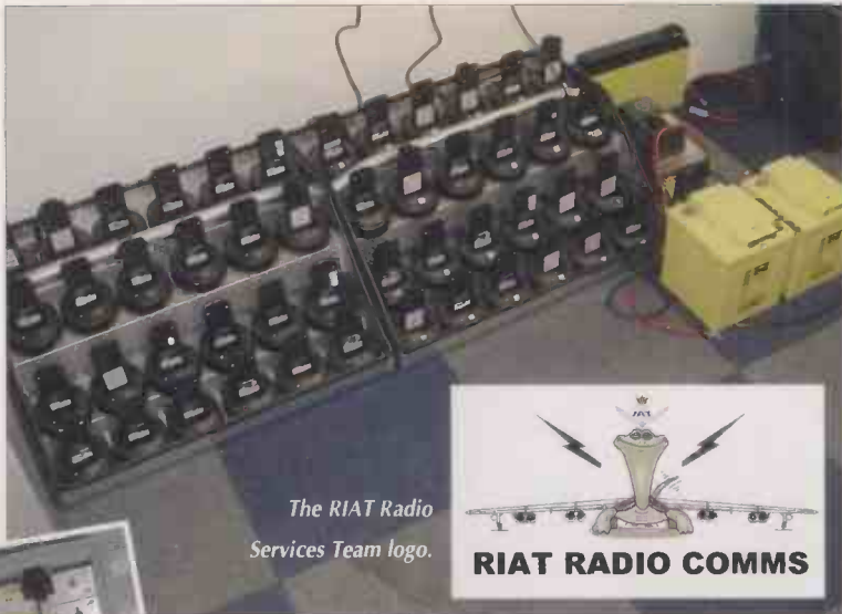
Twelve Phillips/Simoco PRP76 u.h.f. PMR hand portable radios re-packaged into a rack. Receive distribution built into rack. The box top right contains audio isolation transformers. All audio is brought out onto RJ45 cables, which run to PC soundcards.
