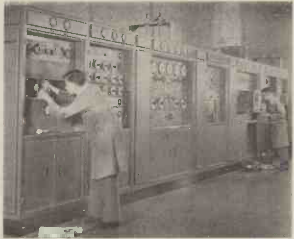
One of the Radio New Zealand transmitters, situated at Titahi Bay, Wellington, N.Z.
