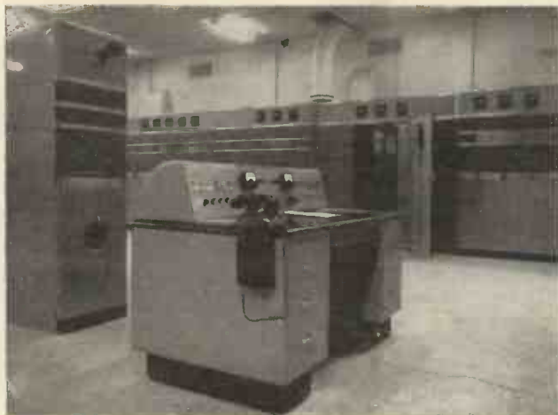
The 50-kW RCA transmitter for VLC, Radio Australia, with monitoring equipment and control desk in the foreground.
