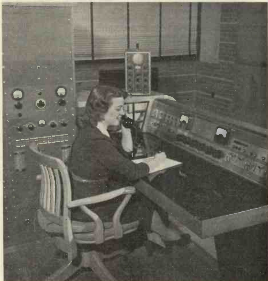
Close up of the main operating console for control of the various sets in the CBC transmitter hall at Sackville, New Brunswick.
