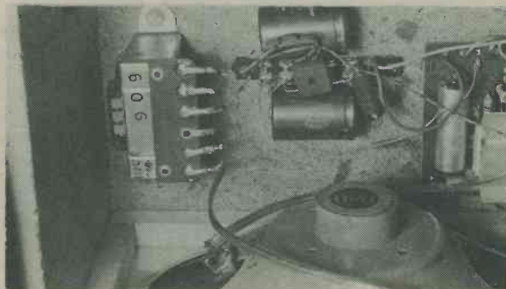
Close-up view of the mains transformer and power supply components
