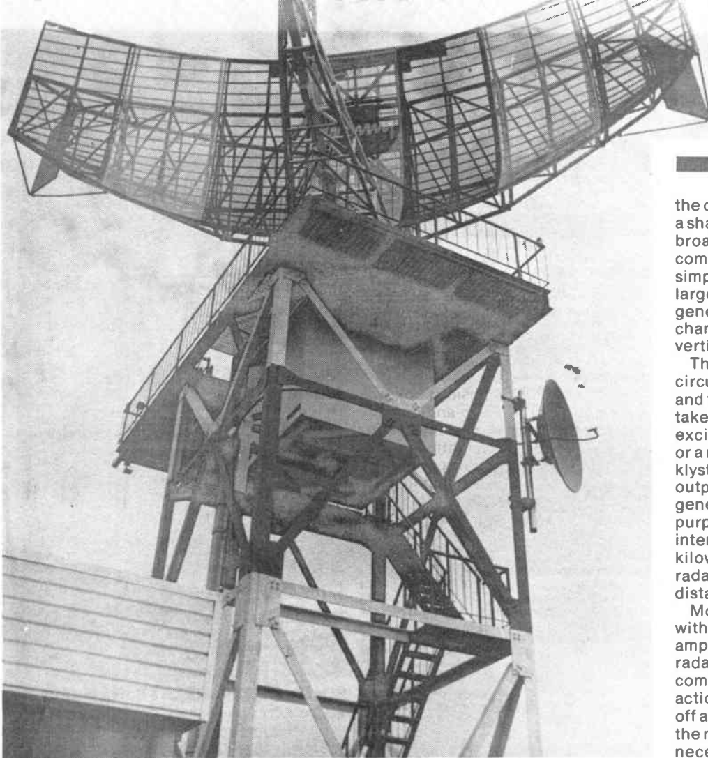
A Plessey AR5 23cm surveillance radar. The microwave dish is part of a link to feed the output of the radar to the air traffic control centre at the opposite side of the airport. This installation is at Bandar Seri Begawan airport in Brunei
