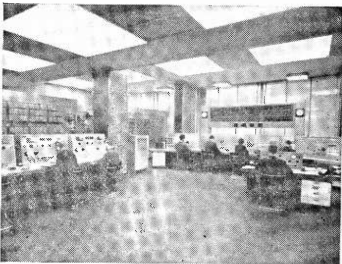
The sound control room of the new Broadcasting House extension in London. This room houses the Technical Operations Supervisor's desk (on the right) and the Main Control desk.
