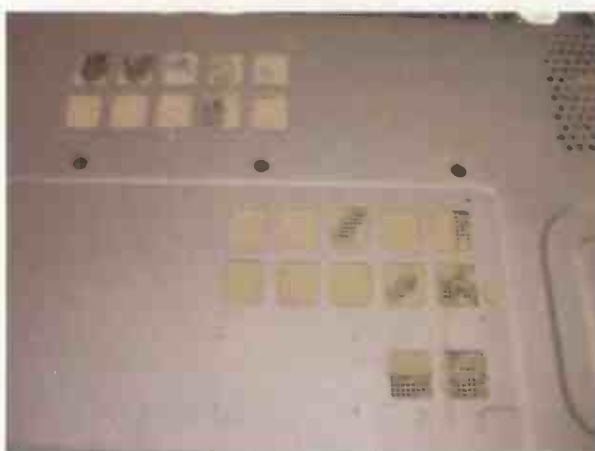
Ventilation blocked, as the back of the panel hasn't been cleaned this can lead to the unit over-heating
