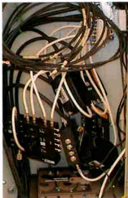
Photo 1: Part of a poor satellite distribution system that had to be rebuilt.
