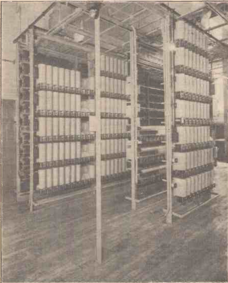
A bank of final selectors.
