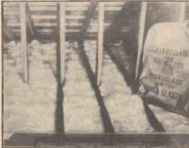
Close-up view of the rafters of a building, showing thermal insulation by means of a glass-wool layer.
