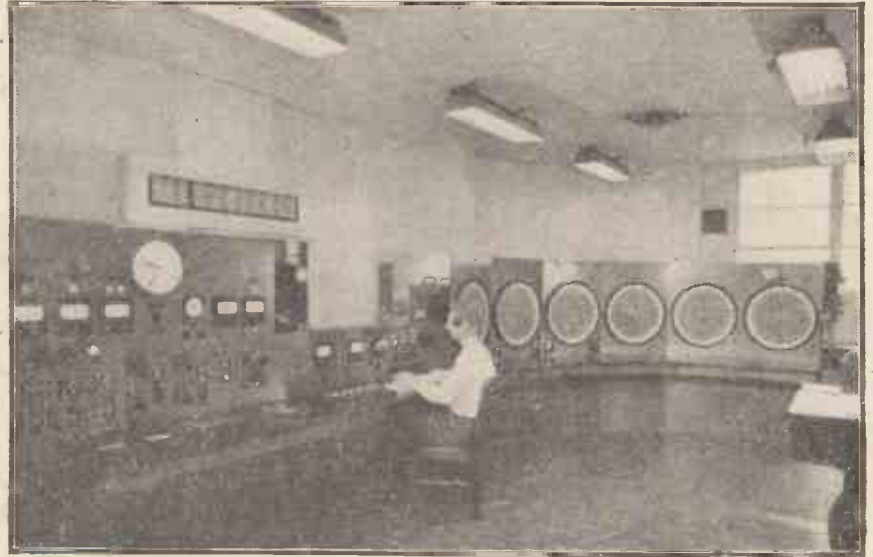
Fig. 9.—Control room of the Convoir tunnel.
