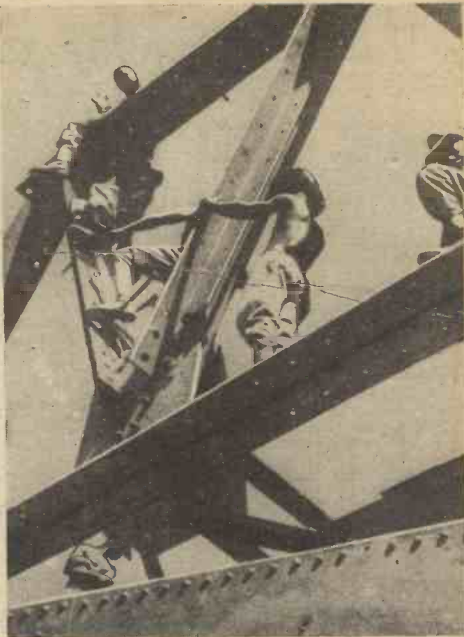
Repairing one of the spans on Pinyinana Bridge, much of the work being done at a considerable height.
