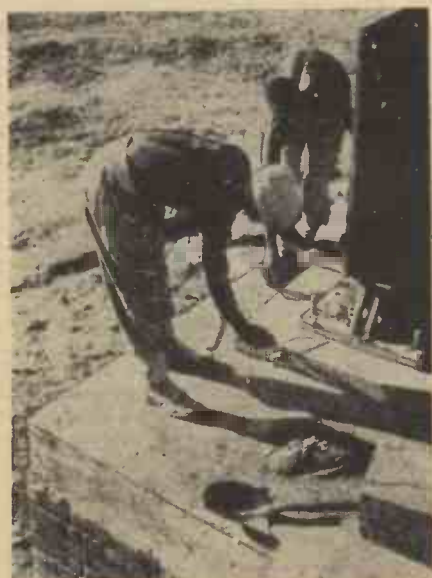
Two sappers from East Africa concreting the base of one of the large piers.
