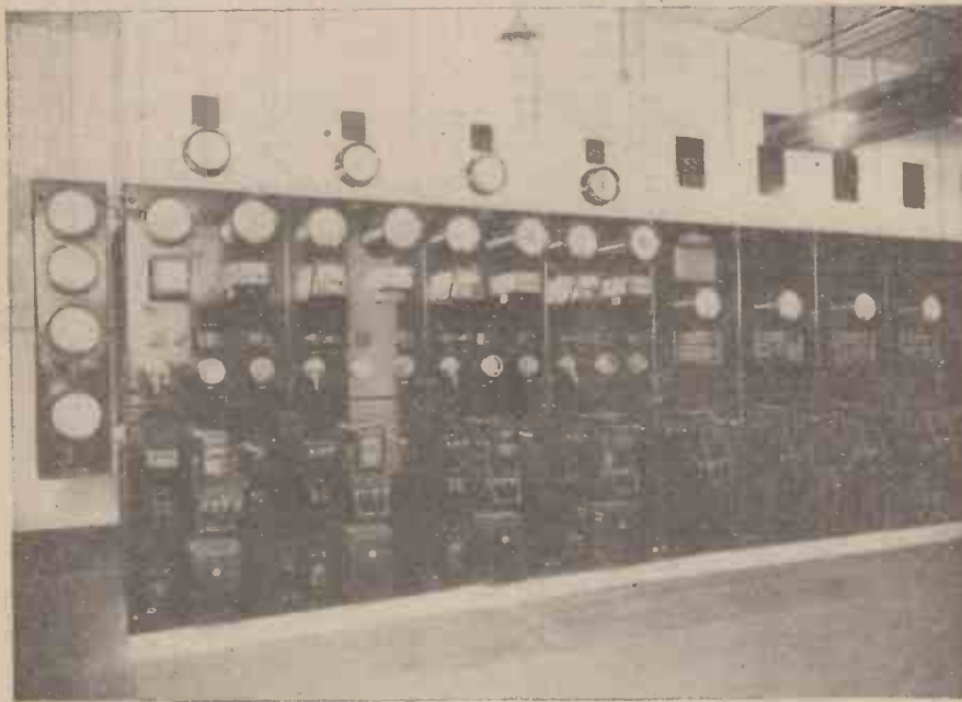
Nine-panel switchboard; at the extreme left is the hinged panel for the synchroscope then the four generating-set panels; and on the right the five feeder panels for the building.
