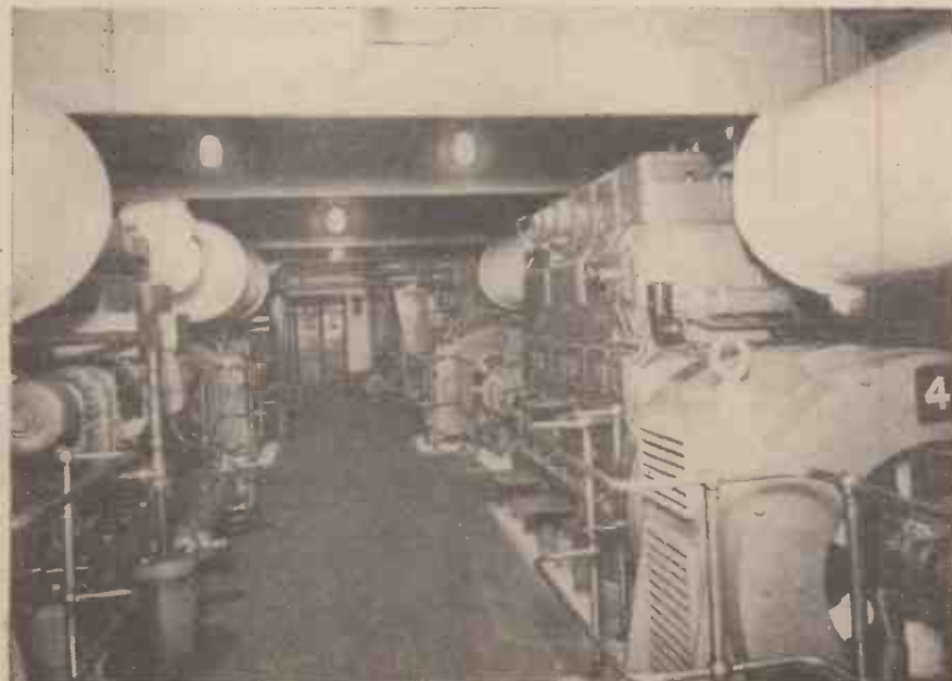
General view of the four 250 kW. Petter engine generating sets at the Horseferry Road Citadel. The two Heenan and Froude coolers are in the background.
