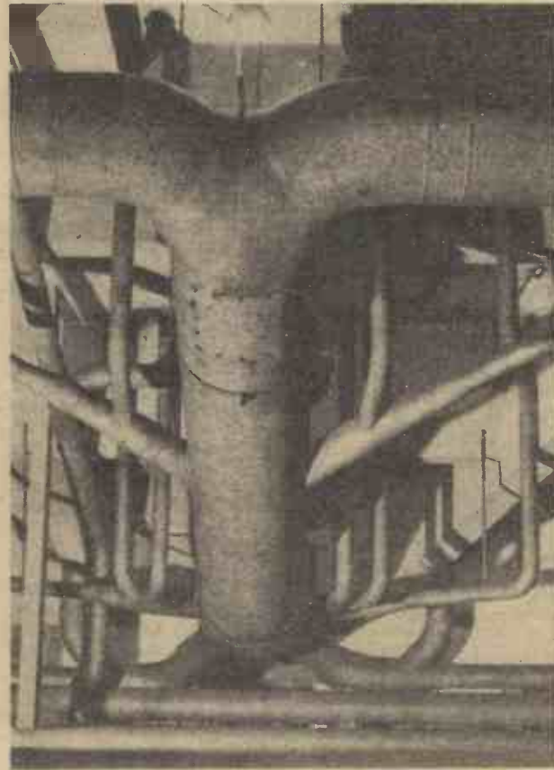
Down in the depths at the County Hall is installed one of the finest air-conditioning plants in the world. Huge pipes start their journey to supply clean, warm and fresh air to the council chamber.
