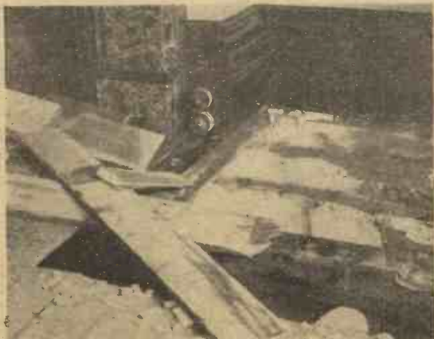
The havoc of dry rot. Showing a room floor completely disintegrated by dry rot infestation, the white fungus of the rot thickly covering the floor joists.
