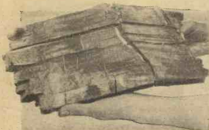
A portion of a wooden floorboard in an advanced stage of dry rot. Note the cracks and fissures in the wood, and the dry, powdery nature of the timber.
