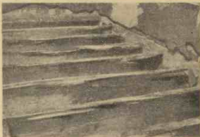
Roof joists which have been rendered completely useless by dry rot.
