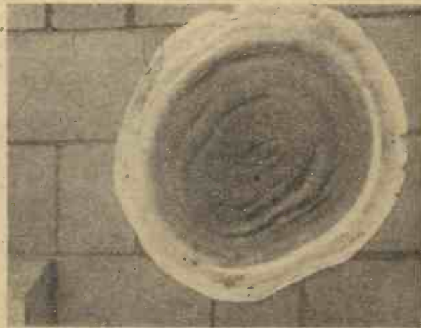
A perfect example of the pancake-like "flower" of the dry rot fungus. In this example, filaments of the fungus have actually penetrated the mortar of the brick wall from infected woodwork behind and have given rise to the mature "flower" form of the fungus, which, from its convoluted surfaces, scatters countless millions of seeds.
