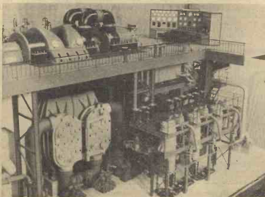
Fig. 3.—The water system showing the large pipes—left foreground—which admit circulating water to the condenser.
