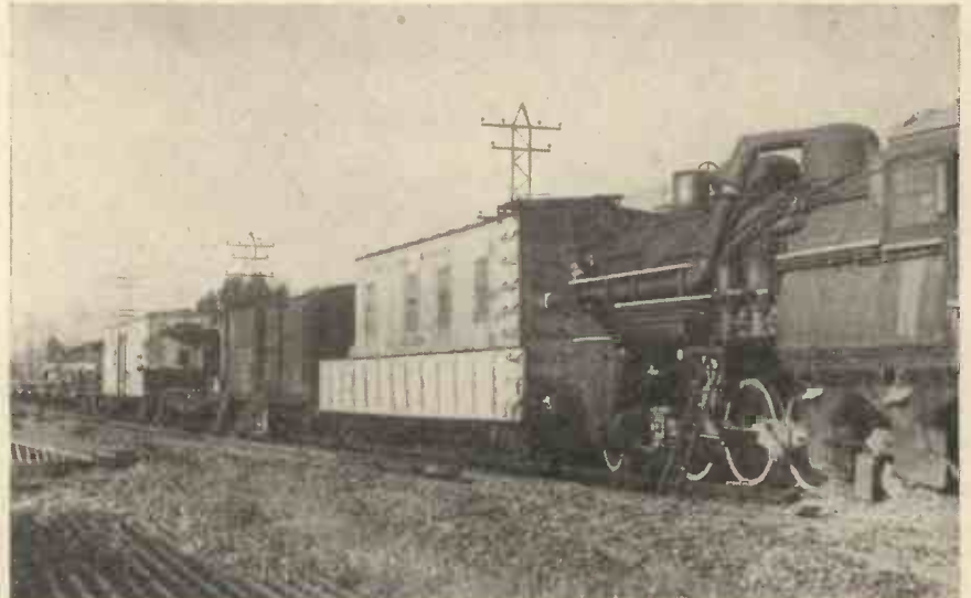
In the Sperry Mobile Welding Unit, a locomotive supplies steam to drive two powerful turbo-generators which provide current for welding machine and auxiliary equipment. Behind the generator is a supply car, next comes a rack car carrying standard rail, followed by the welding car and a string of flat cars.
