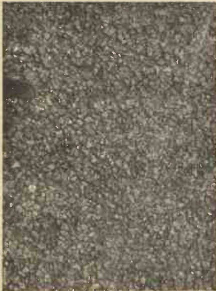
A modern macadamised road surface composed of small stones welded together that the foundations are kept absolutely waterproof.
