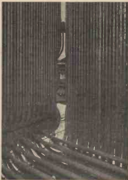
In a modern boiler water tubes line the furnace walls in every direction.
